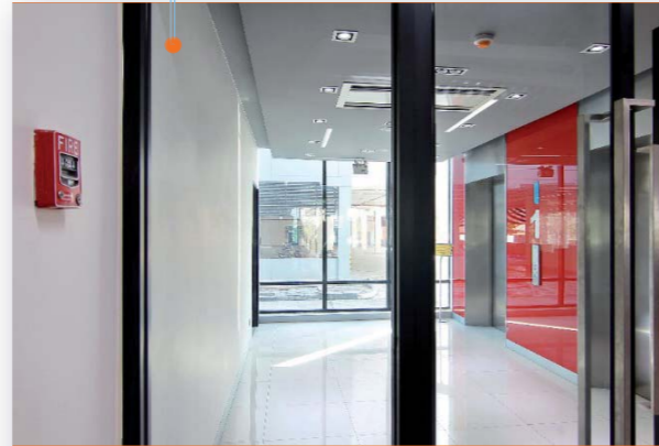
Fire Alarm System
