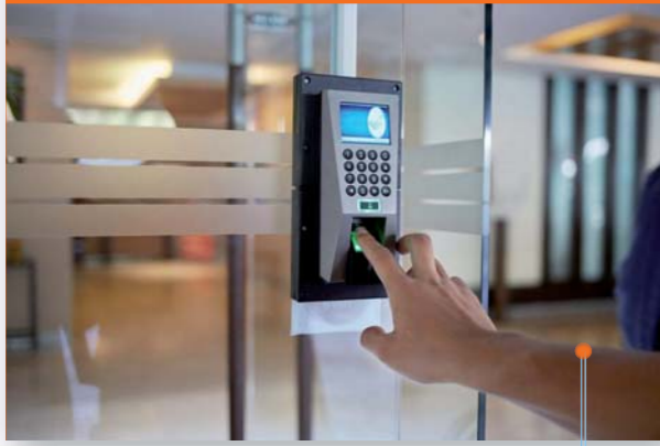
Access Control System
