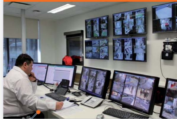
Building Management System
