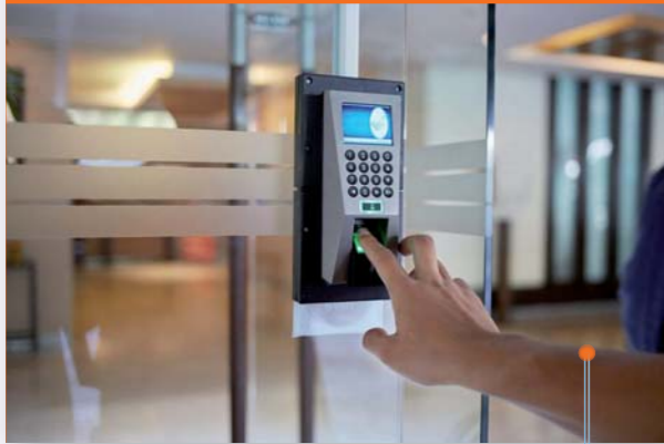
Access Control System
