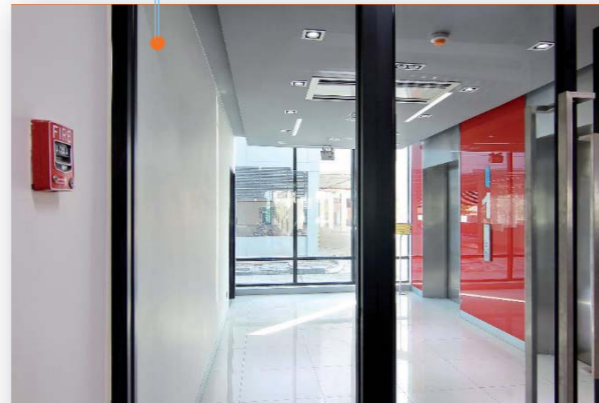
Fire Alarm System
